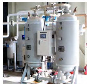
Dryer for low pressure air
