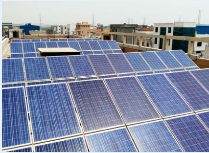
Solar panels on the roof of the Gerresheimer Triveni plant
